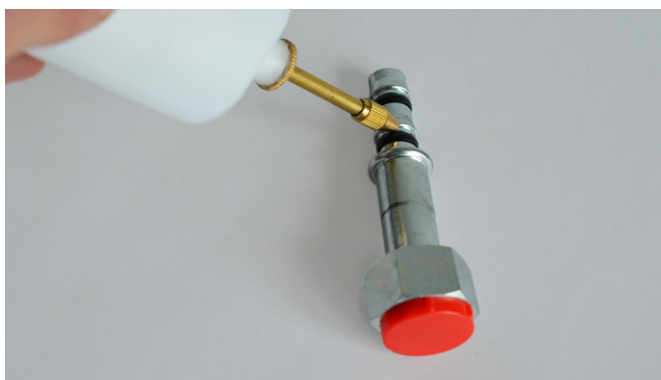
5 Grease the end of the fitting with the same oil used in the air conditioning system
